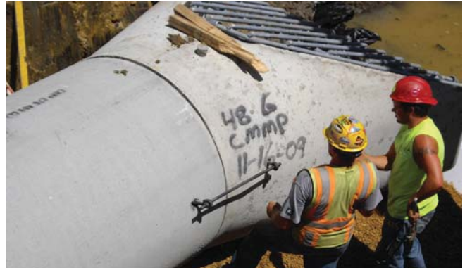
REEDSBURG, WI, FLOOD RECOVERY & MITIGATION
